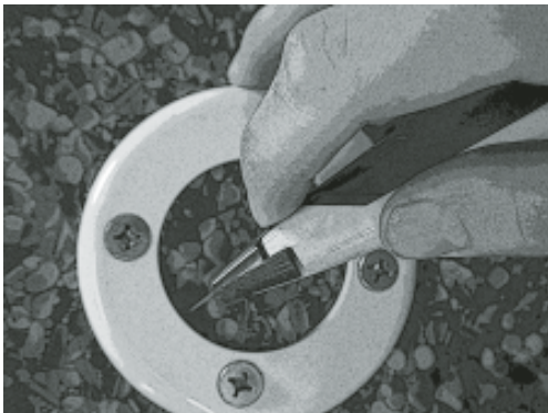
Trim liner from return opening.
