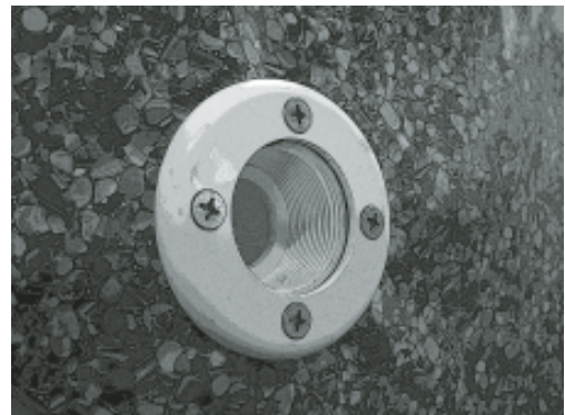
Return faceplate installed.
