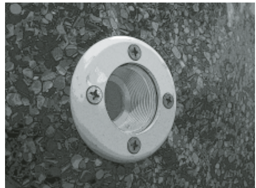
Return faceplate installed.
